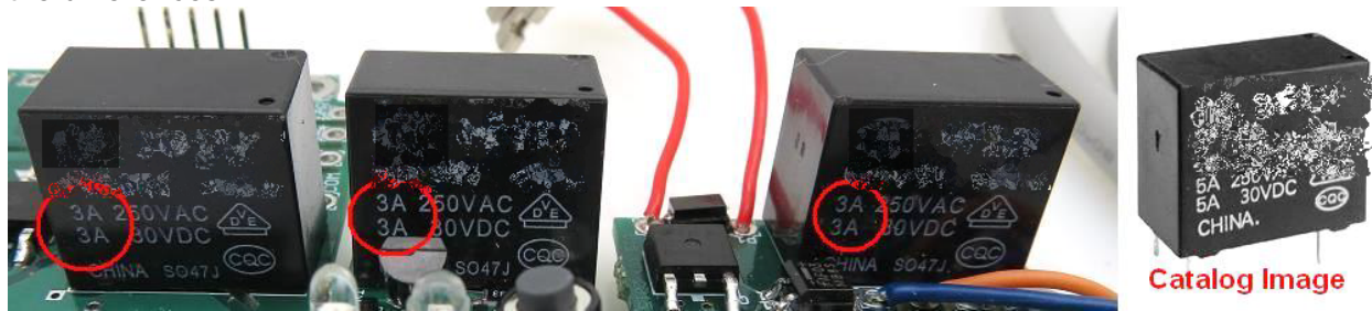
Figure 6: Left is the relay on a “New” P-1-Small Rev. 2C board; 2 nd from the left is a Switch-1 (SW-1) relay; 3 rd from the left is a Small Split Slender relay; and extreme right is a copy of the catalog image of the relay. Note the current rating differences at 250VAC between the left relays and the catalog relay.
